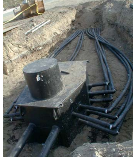
Ground source manifold. The loop field contained over 300 bore holes.
