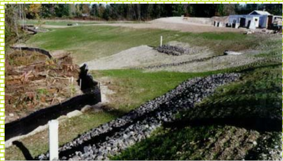
A system of level spreaders allowed surface water to infiltrate the site more naturally. This allowed a wetland downslope of the Sakai Intermediate School, Bainbridge Island, Washington, to be fed rather than starved for water.
